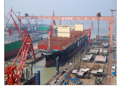
MSC Tessa under construction at Hudong-Zhonghua Shipbuilding. With a carrying capacity of 24,116 TEU, MSC Tessa will surpass Evergreen's Ever Alot by 112 TEU to take the title of world's largest Con.
