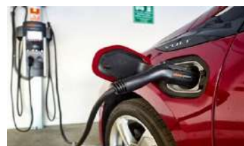
EV charging station
